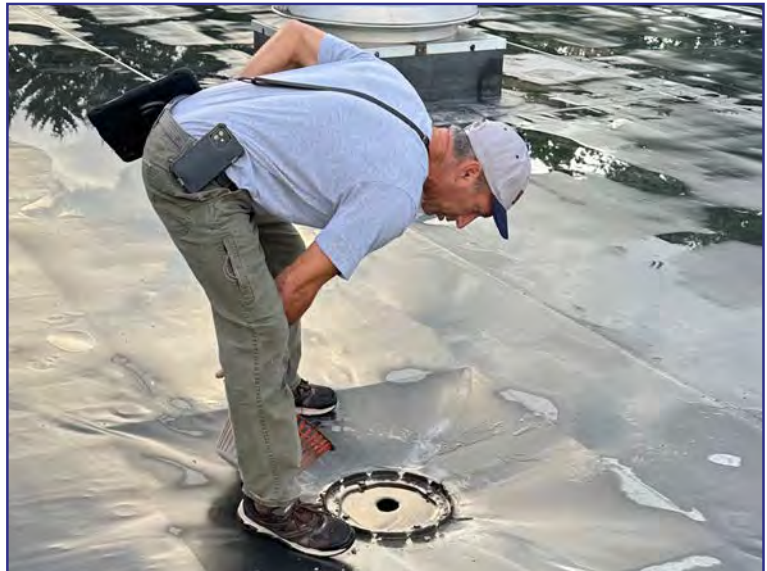
The warranty inspector observing a new drain in action just after a large rainfall
